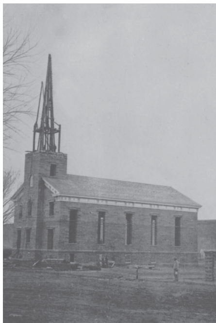
The St. George Tabernacle under construction, date unknown. Photograph courtesy Utah State Historical Society.
