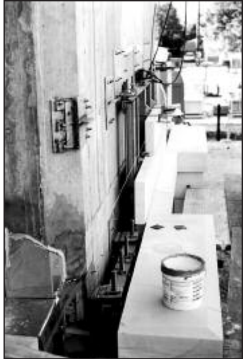
Photograph showing the limestone “vener” panels being attached to the steel frame, August 2001. The finished stone sections were first attached to steel frames, then the frames were attached in sections to the concrete shell. Photograph courtesy of Roger P. Jackson.
