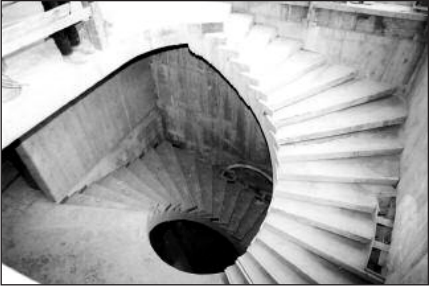
Circular staircase under construction in the southwest corner of the building, July 2001. Photograph courtesy of Roger P. Jackson.
