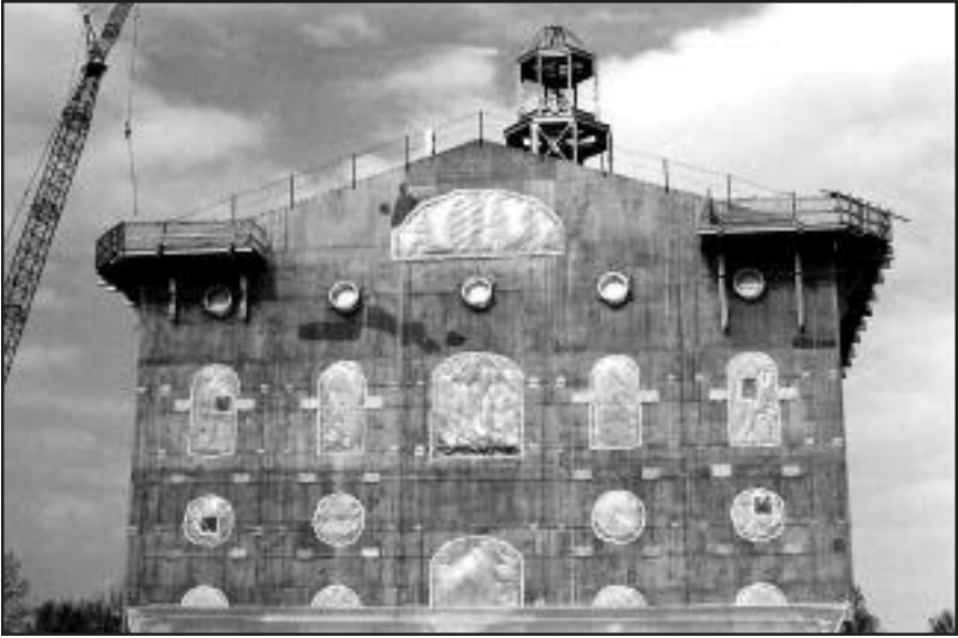
Concrete shell of the Nauvoo Temple, east side, April 2001. Photograph courtesy of Roger P. Jackson.
