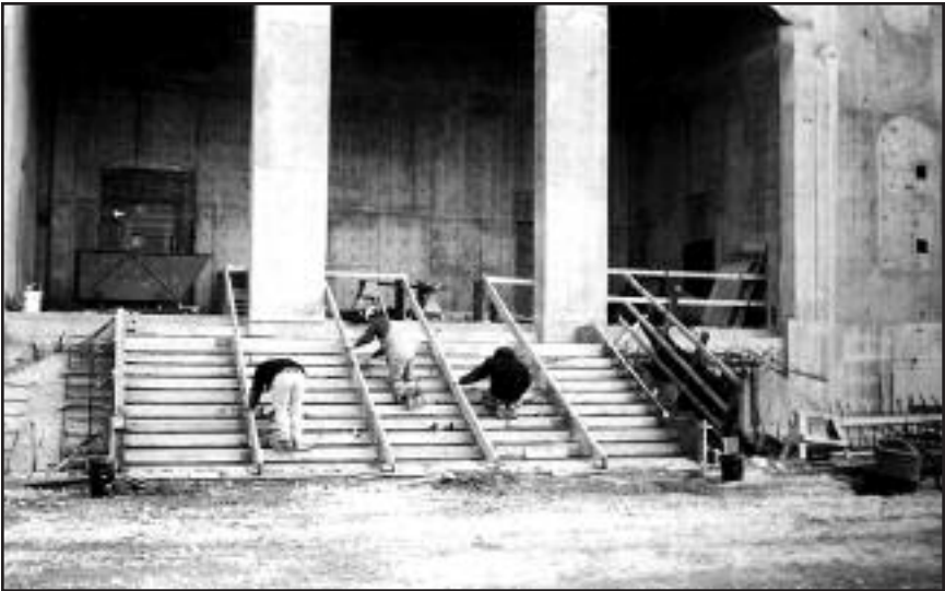
Workers preparing to pour the concrete for the front steps, February 2001. Photograph courtesy of Roger P. Jackson.
